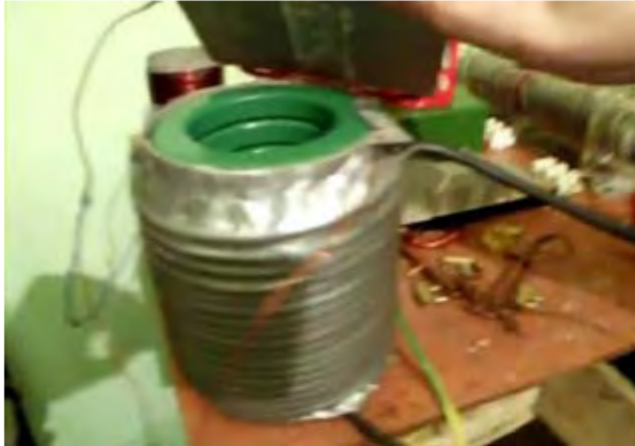
Figure 112: Isolation transformer. See above.
